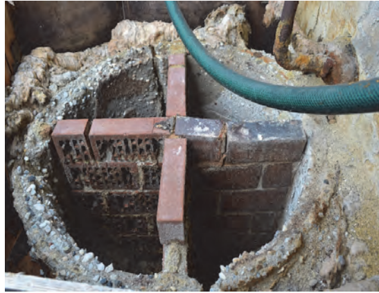
Fig. 4. Destroyed elements of concrete exhaust gases silencer – corrosion effect of acid gases from the engine
